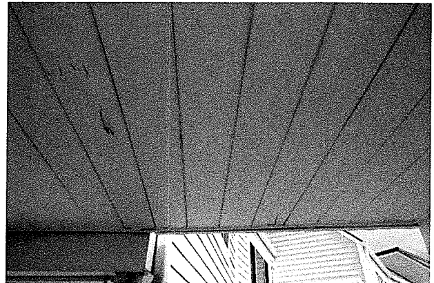
P 96: Damage Ceiling Panels, Elevated Walkway
