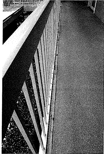
P 106: Rusted Steel
