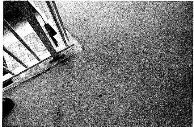
P 100: Rusted Steel & Concrete Crack, Elevated Walkway
