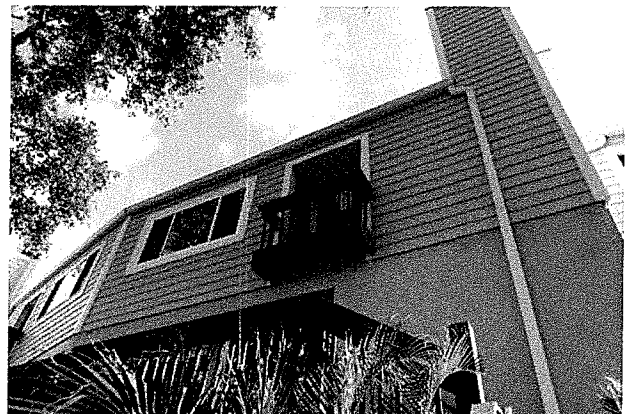
P 28: Uncoated Wood at Balcony, South Elevation
