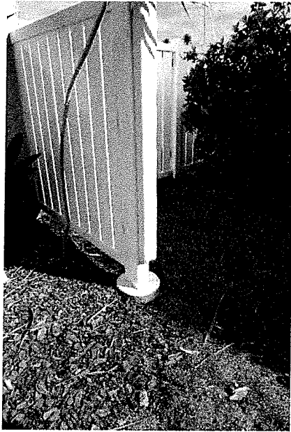
P 9: Rusted Fence
