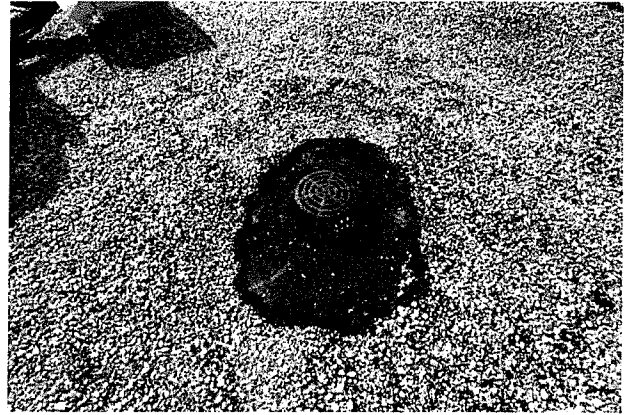
P 50: Rusted Drain
