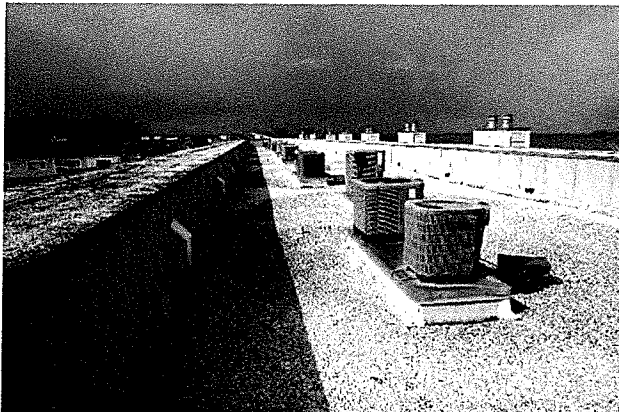
P 47: North Building Roof, A/C Units
