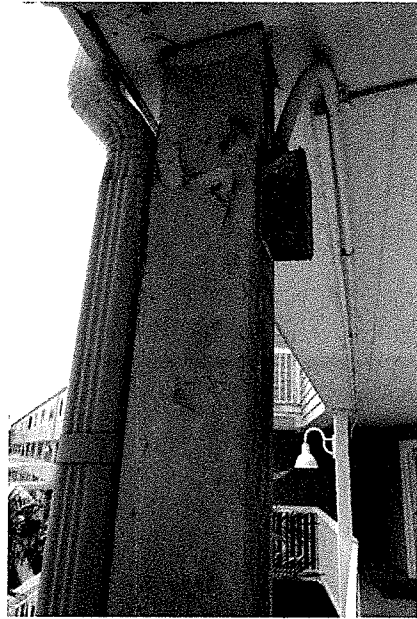
P 98: Rusted Support & Deteriorating Coating, Elevated Walkway
