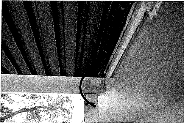
P 37: Rusted Steel underneath Walkway; North Elevation, South Building
