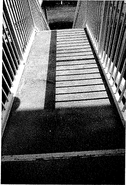
P 105: No Coating on Stairwell Walkway
