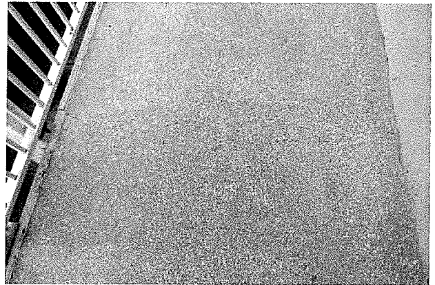
P 88: Concrete Crack, Elevated Walkway
