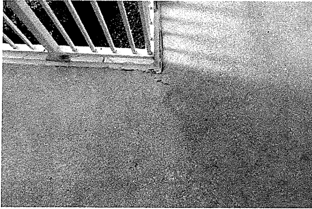
P 93: Concrete Spall, Elevated Walkway
