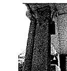
P98 RUSTED SUPPORT & DETERIORATING COATING, ELEVATED WALKWAY
