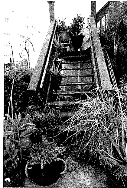
P 12: Deteriorating Wood Stairwell, West Elevation
