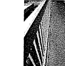
P106 RUSTED STEEL
