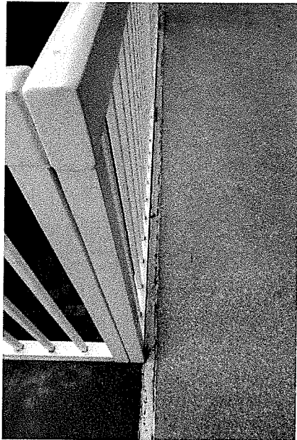
P 87: Rusted Steel, Elevated Walkway
