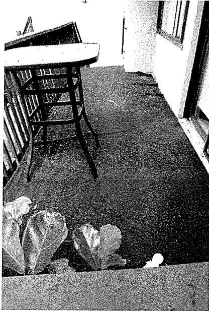
P 69: 2 nd Floor Balcony & Rug, Unit 30
