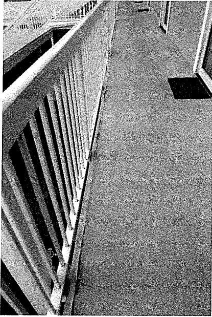
P 89: Rusted Steel, Elevated Walkway
