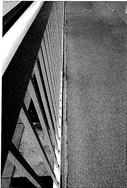
P 103: Rusted Steel, Elevated Walkway
