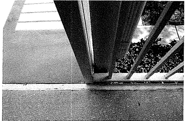
P 108: Rusted Steel
