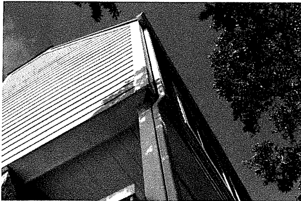
P 35: Missing Wood Beam, East Elevation
