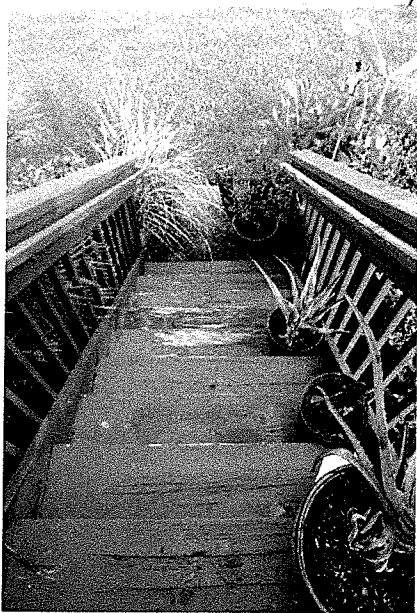
P 13: Deteriorating Wood Stairwell, West Elevation
