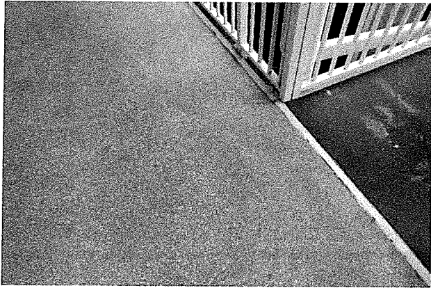
P 85: Rusted Joint, Elevated Walkway
