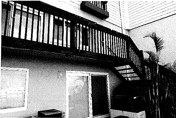
P 19: Deteriorating Wood Railing, West Elevation
