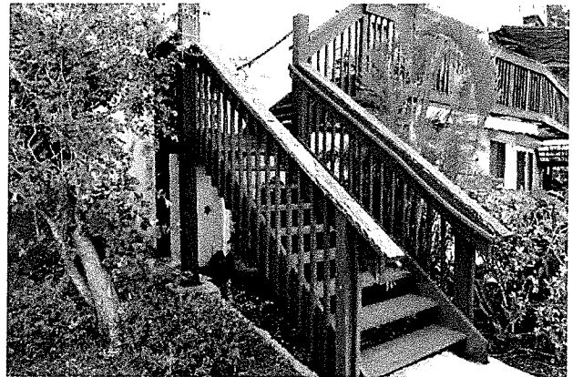
P 24: Deteriorating Wood Railing, West Elevation
