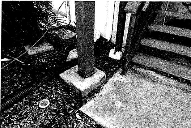
P 27: Rust at Concrete Base, South Elevation
