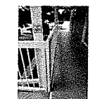
P107 RUSTED STEEL
