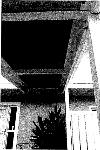
P 5: Rust Underneath Walkway
