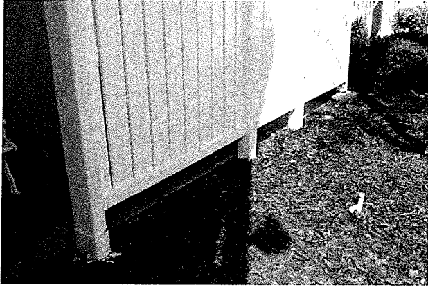
P 41: Rusted Steel Base; North Elevation, South Building
