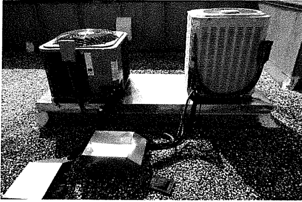
P 49: A/C Units with L-Fasteners
