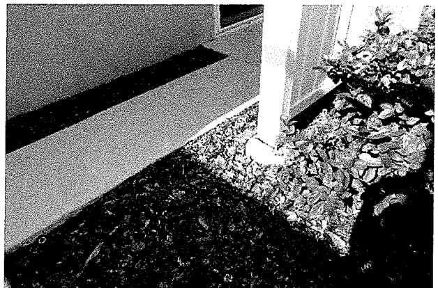
P 40: Rusted Steel Base; North Elevation, South Building
